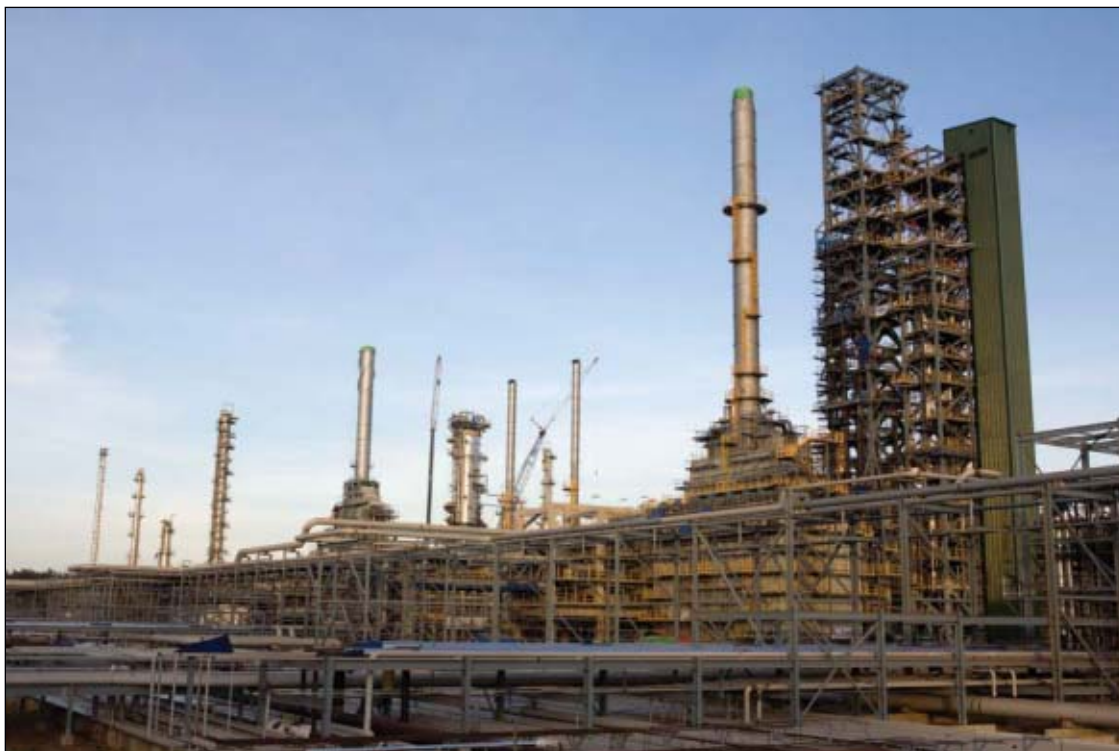
Vietnam opened its first refinery, a $3 billion project designed to meet a third of Vietnam's fuel demand in 2010. The 148,000-b/d plant in Dung Quat Bay will be operated by state-owned Vietnam Oil & Gas Group (Petrovietnam). This is a continuous catalytic reforming unit under commissioning. Photo from Technip, by Patrick Zachmann/Magnum Photos.
