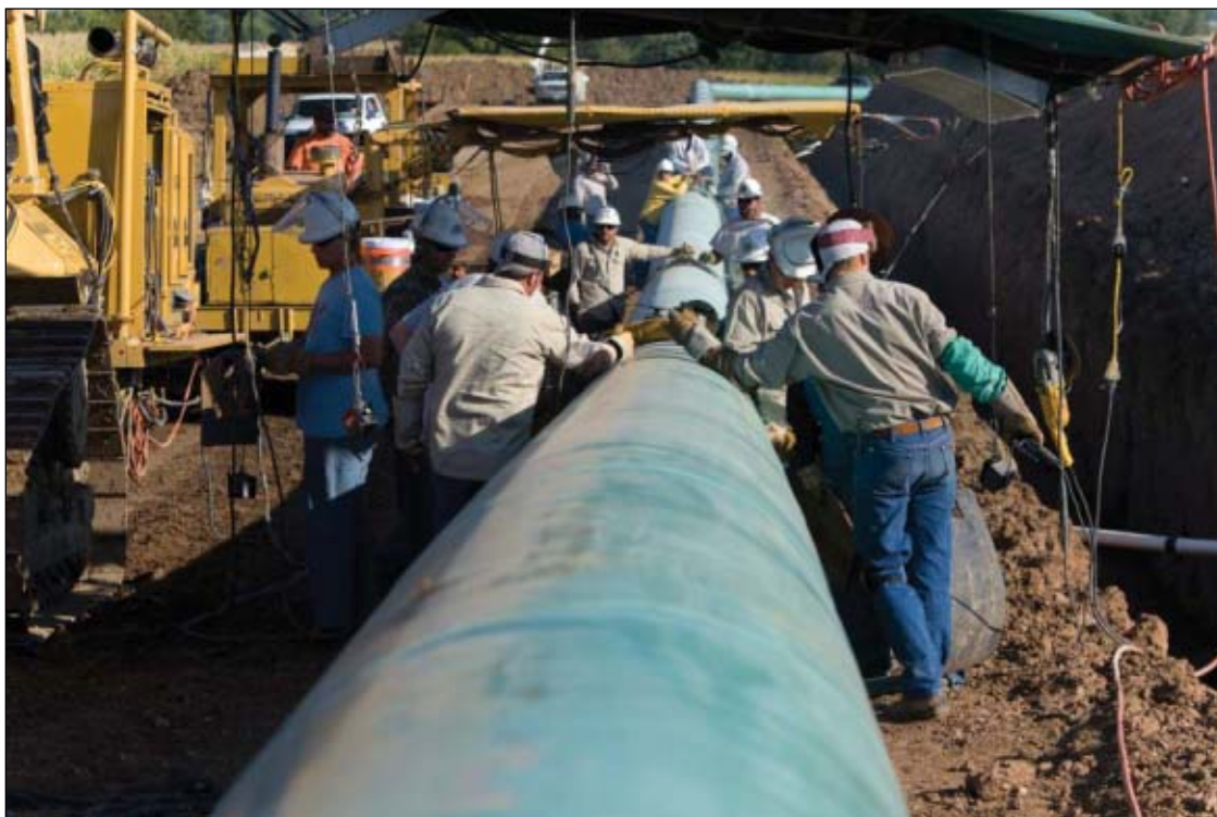
Oneok Partners' 119-mile Guardian Pipeline expansion and extension went into service in February, supplying natural gas to two Wisconsin utilities. Photo from Oneok.
